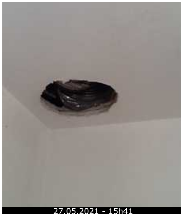
Photo 28 (WC / Ventilation / Manque accessoire(s))
